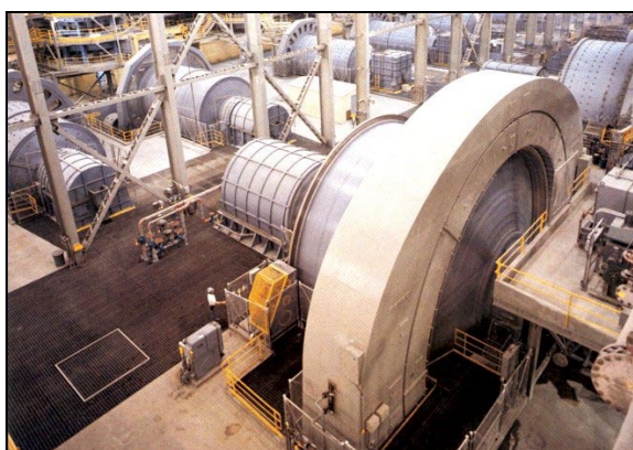
Figure 2.5: Grinding circuit with AG mills (primary grinding, right side) and ball mills (secondary grinding, left side)
