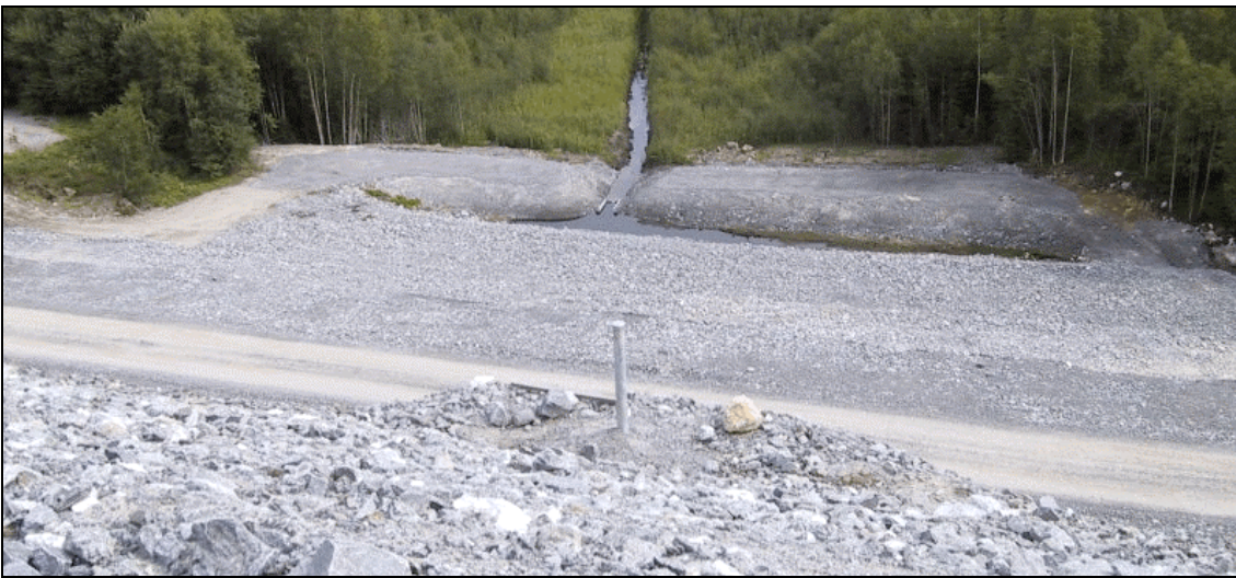
Figure 3.23: Another ditch for collection and flow measuring of seepage water alongside the dam [66, Base metals group, 2002]
