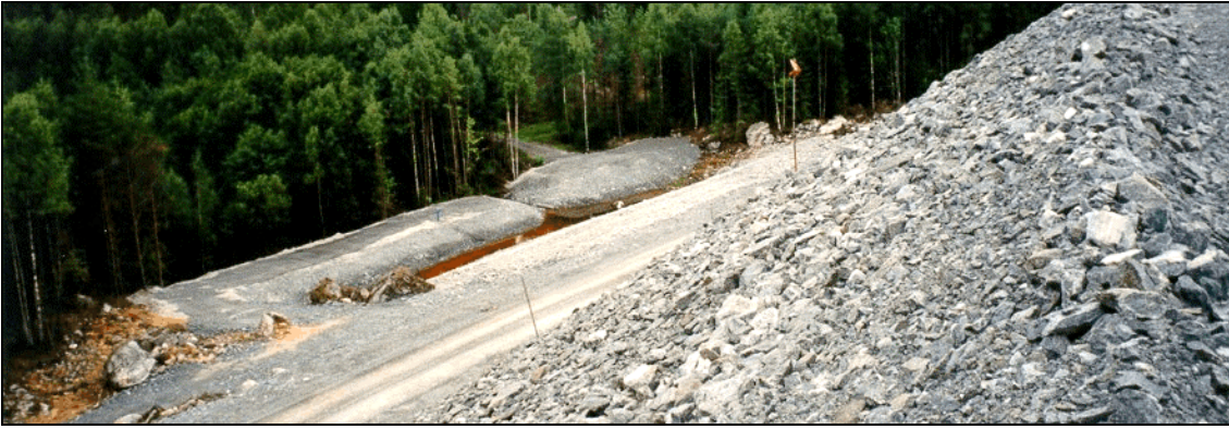
Figure 3.22: Ditch for collection and flow measuring of seepage water alongside the dam [66, Base metals group, 2002]
